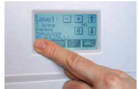
Touch screen on the profi-air ventilation unit
